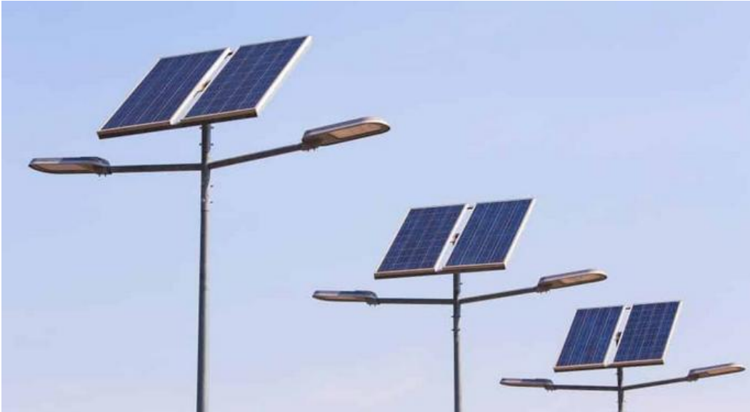
Figure 16. Outdoor lighting (source: https://www.streetlights-solar.com/popularity-solar-outdoor-lighting-us.html )
