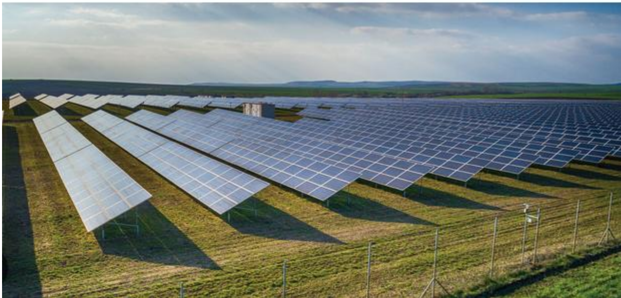
Figure 12. Utility-Scale Photovoltaic Systems Source: energy.mit.edu/news/solar-photovoltaics-the-benefits-outweigh-the-costs/
