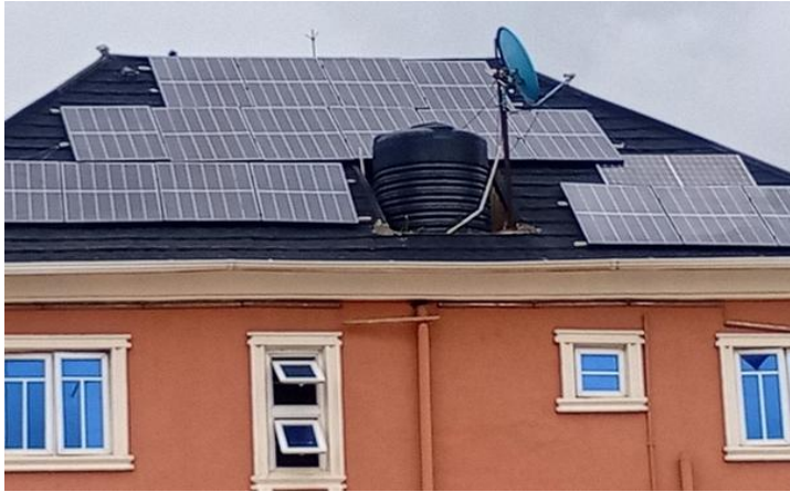
Figure 3. A solar panel on a rooftop in a Nigerian House
