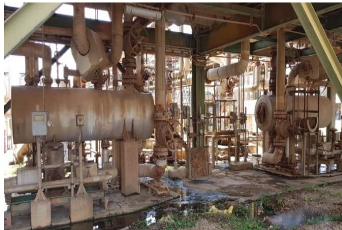
Figure 1. The High-Pressure Heaters
